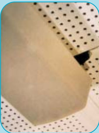
Perforated AIB ceiling tiles
