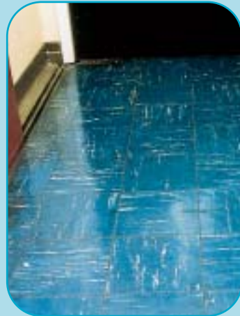
Asbestos-containing floor tiles
